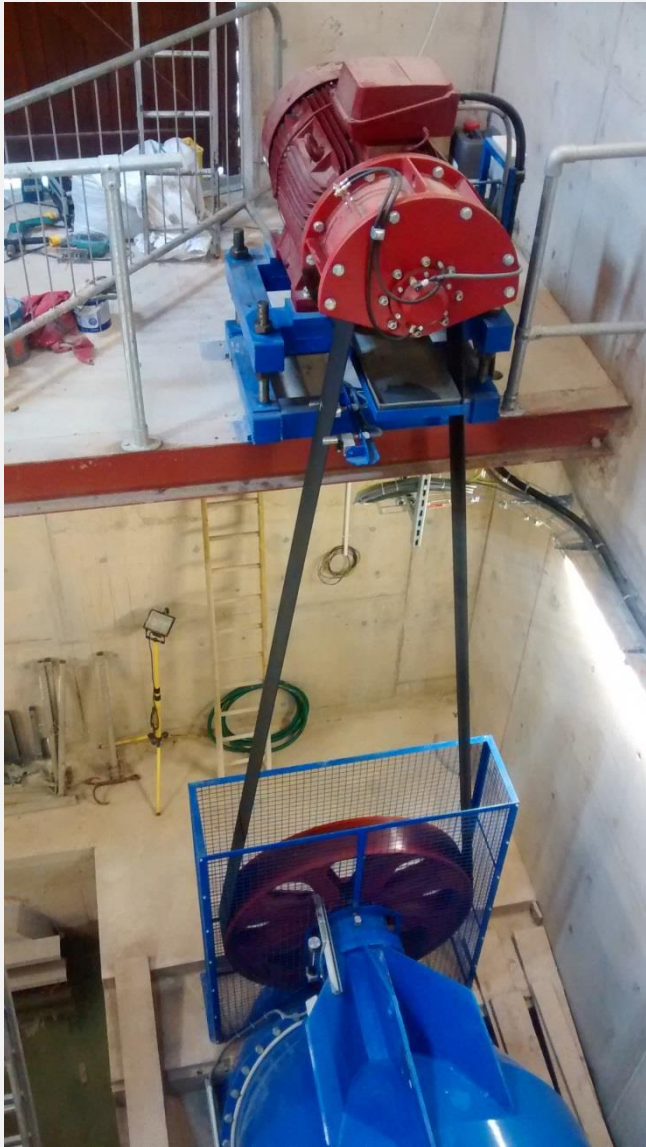
Hydro turbine for local community project
