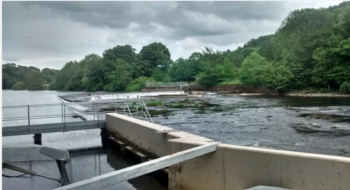
Installations of the micro-hydro power plant
